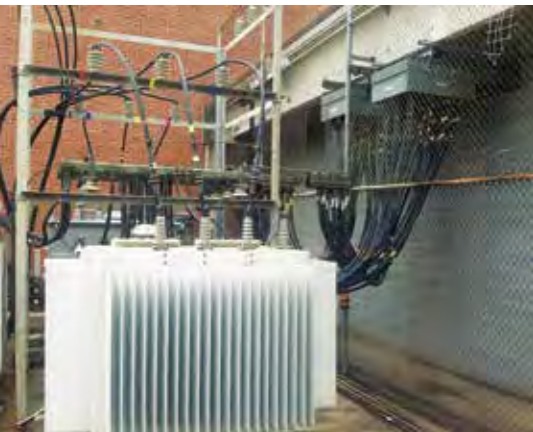
(9) ELECTRIC SERVICE ENTRANCE.
