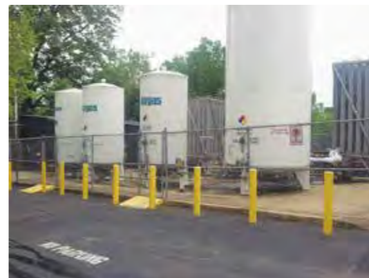
(7) BULK MEDICAL GAS STORAGE.
