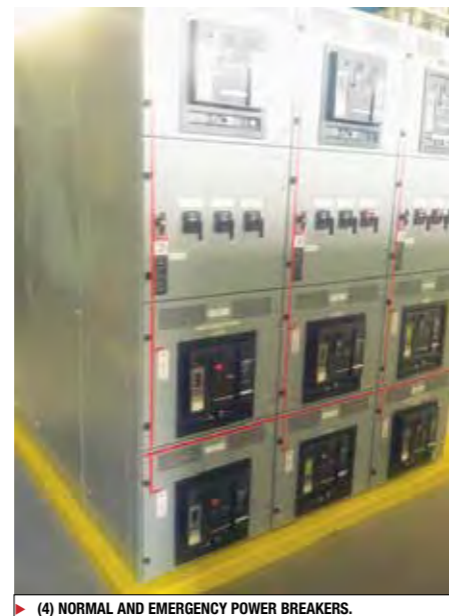
(4) NORMAL AND EMERGENCY POWER BREAKERS.
