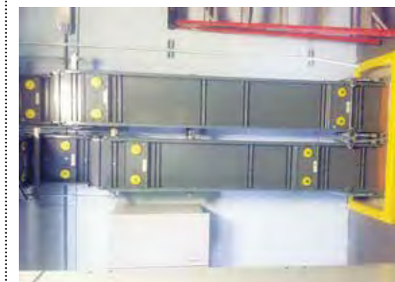
(2) AN ELECTRIC BUSS DUCT.
