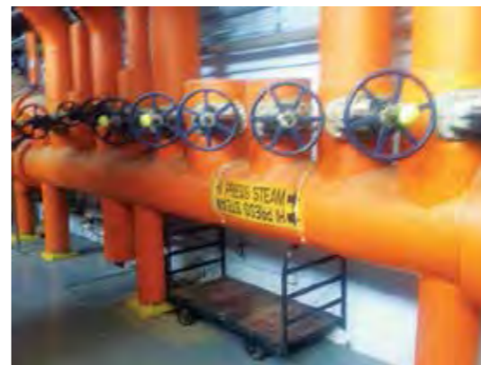
(1) A STEAM HEADER. (PHOTOS BY AUTHOR.)
